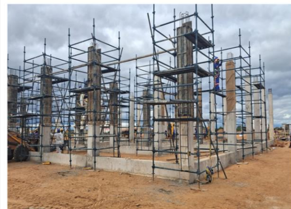
400kV Mmamabula Substation project (Botswana)
