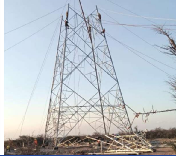
400 kV D/C Transmission Line TaZa Project (Tanzania)
