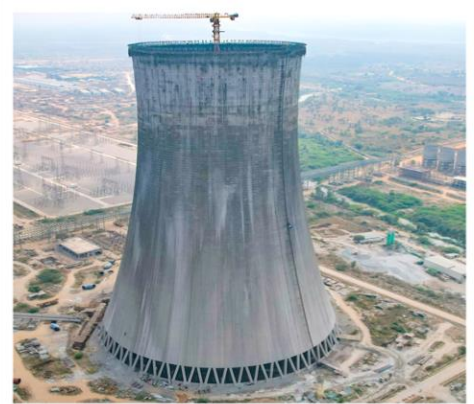
Cooling tower at Udangudi and Yadadiri
