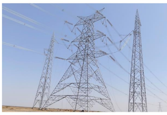
765 kV D/C Transmission lines in Khavda, Gujarat
