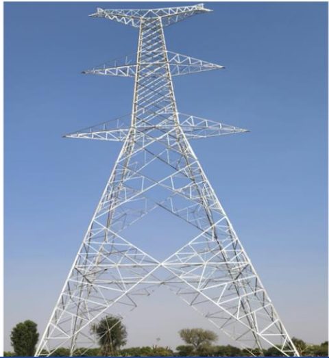
Koppal-II PS – Narendra (New) 765 kV D/C line
