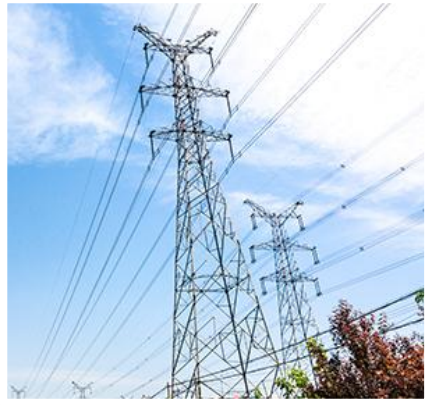
Power Transmission Lines
