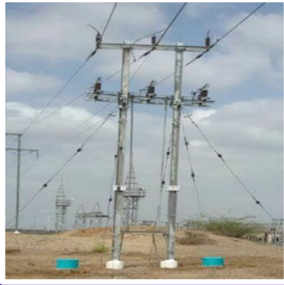
Power Distribution Network Establishment
