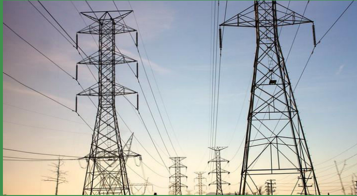
02 Power and Transmission
