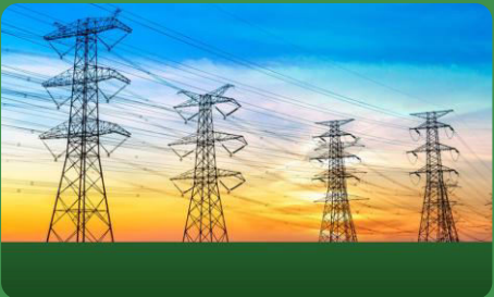
Transmission Line Tower
