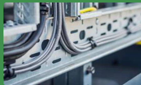
Cable Tray & Earthing Material
