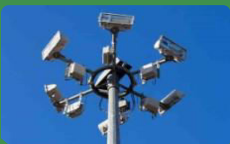
High Mast & Lighting Pole
