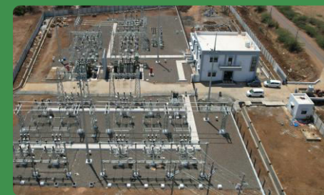
Pooling Sub-Station Development
