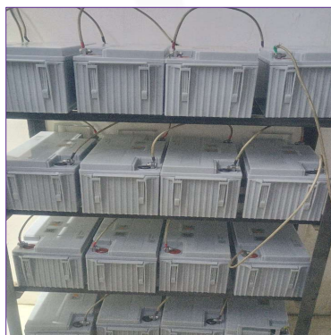
UPS battery recycling
