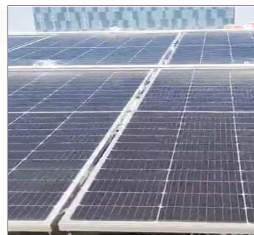
Rooftop solar installations
