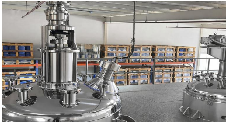
Saudi Arabia Chemical Blending Facility
