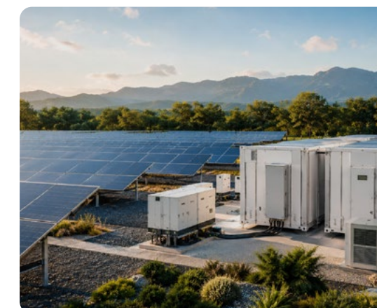
Solar and energy storage
