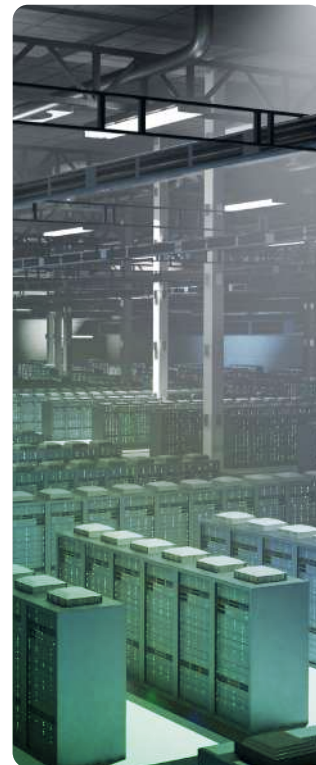
Data Centre Building
