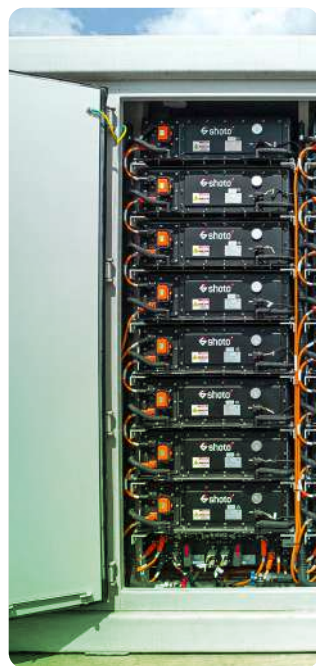
Container Manufacturing (including battery containers for data centre applications)
