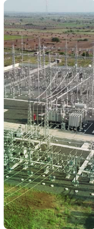
Pooling Sub-Station Development
