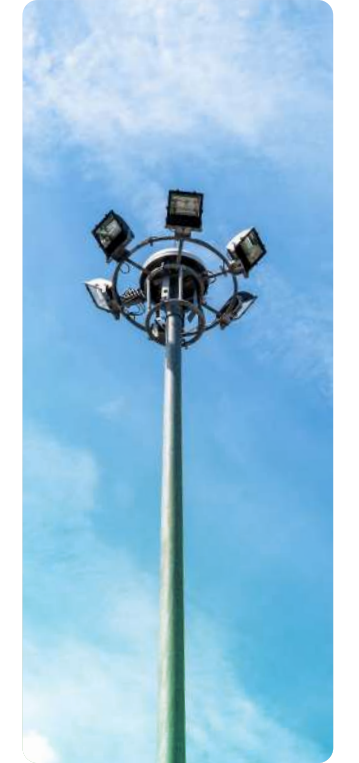
High Mast & Lighting Pole
