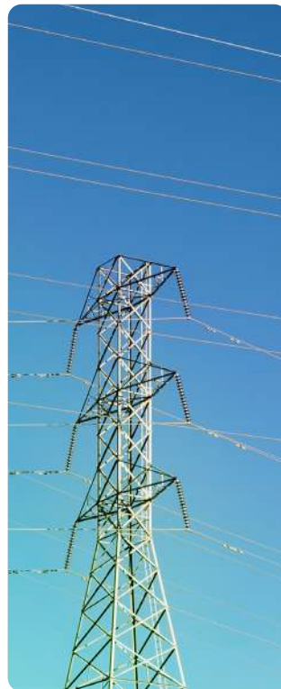
Transmission Line Tower
