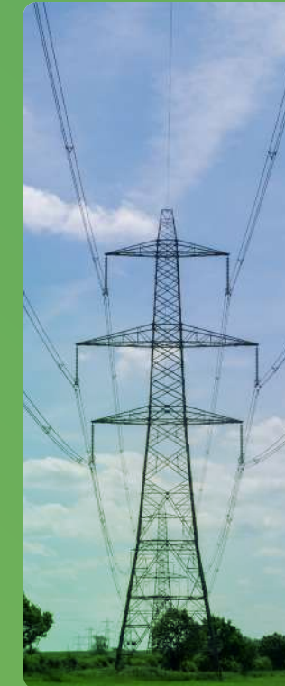
Power and Transmission
