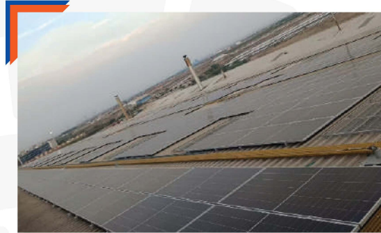
Kandla Plant (Capacity: 600 KWP)
