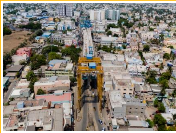
Chennai Metro [RMC supply]
