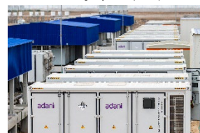
3.55 GWh BESS at Khavda, Gujarat
