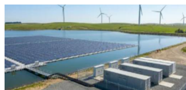
BESS for Renewable Energy Integration
