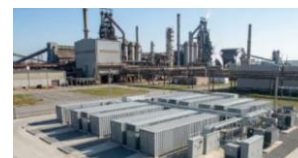
BESS for Industrial Application
