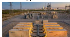
Transmission & Distribution Deferral BESS
