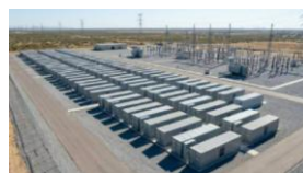
Grid Scale BESS
