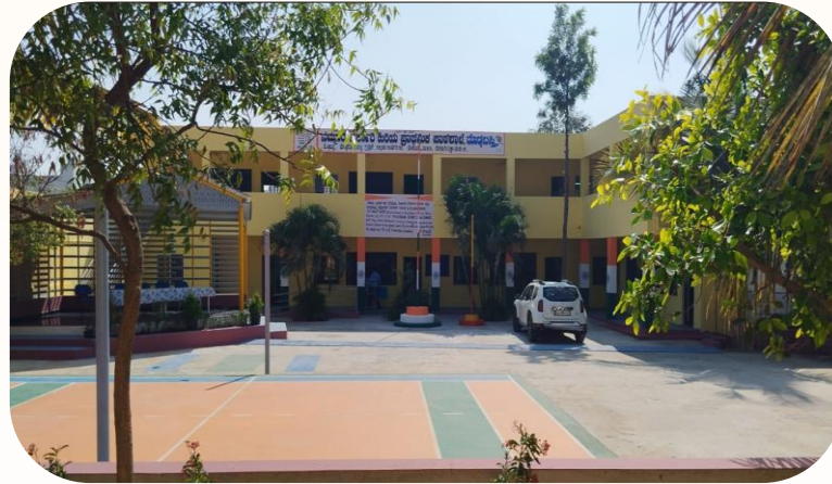
Construction of new class rooms, compound wall, PCC for playground, seating arrangements, podium the events in Govt. Primary School, Doddabasti
