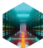
Telecom & Data Centers
