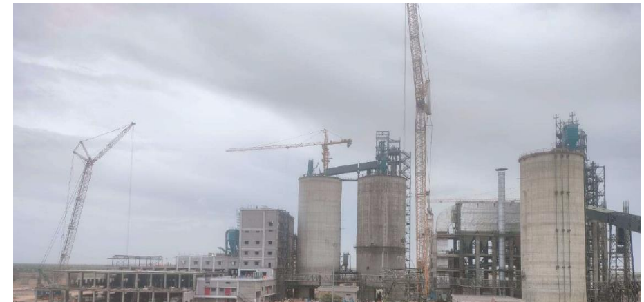
Nagaur IU – cement grinding, packing & dispatch
