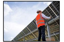
Solar Mounting Structures
