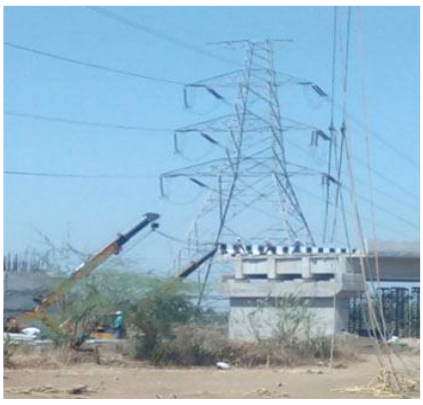
Modification And Upgradation Of System
