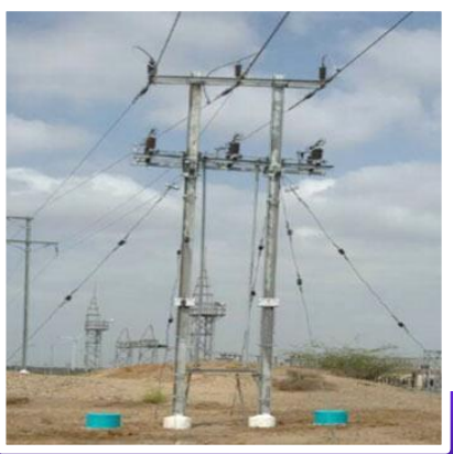
Power Distribution Network Establishment
