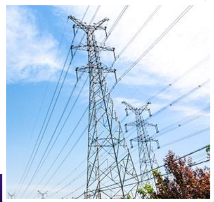
Power Transmission Lines
