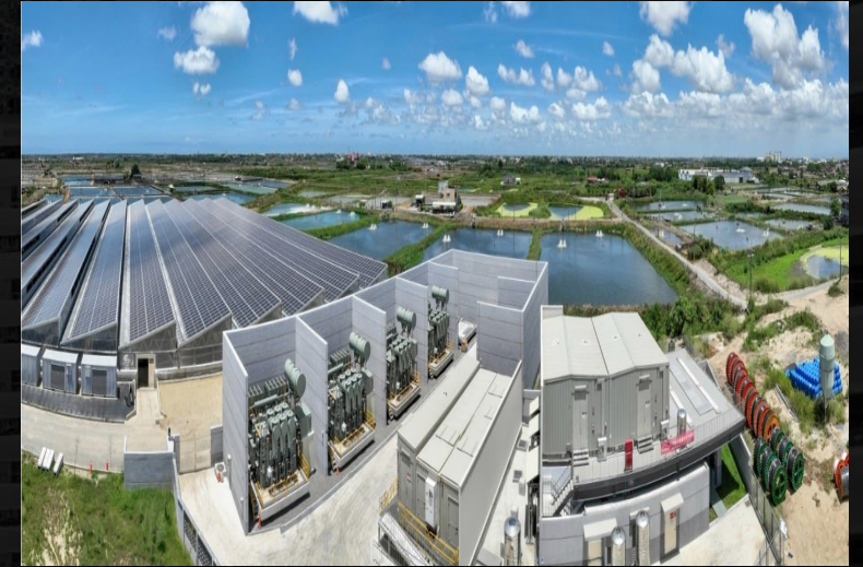
Load Pooling Station and Main Pooling Station, comprising 56 bays of 400 kV GIS and 12.8 km of 400 kV GIB for 100 GW solar park in western India
