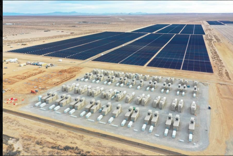
First Battery Energy Storage project of 165 MW/330MWh at Hebbatam, Andhra Pradesh
