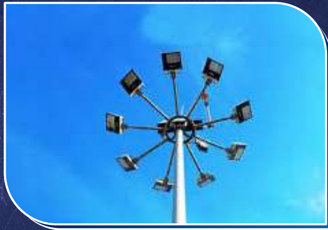
High Mast Lightening Poles
