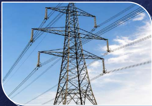
Transmission Line Towers
