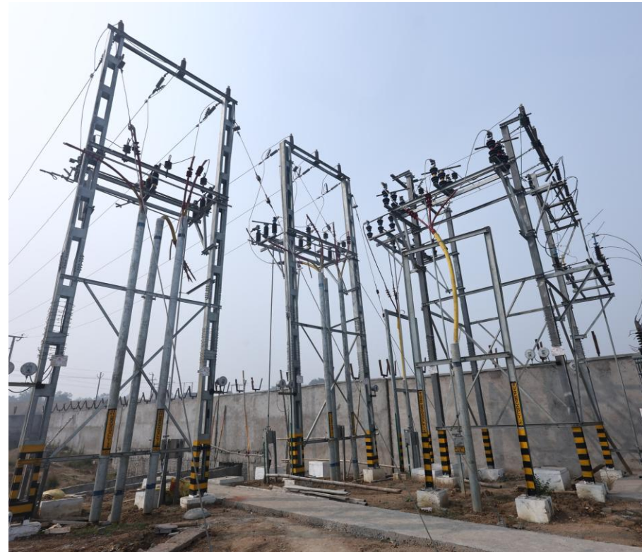
33/11kV Substation featuring 2x8 MVA transformers with TPCODL in Odisha Status: On-going Substation: 9 (no.) Line Length: 192 Ckm HT
