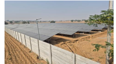
Solar Power Plant 3 Hisar, Haryana
