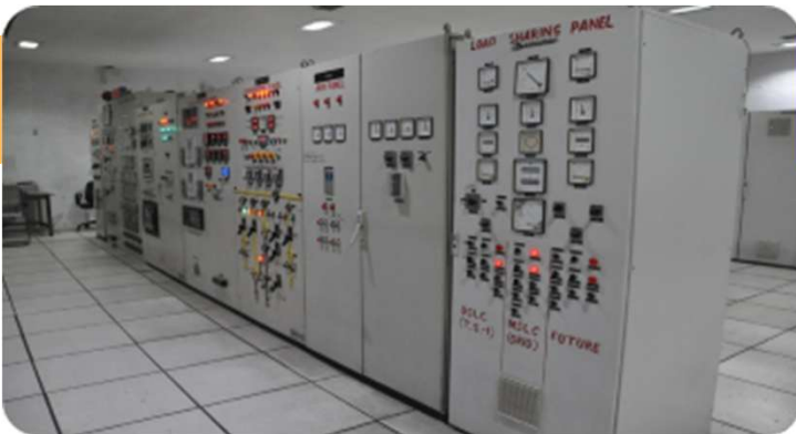
Cogeneration control panel
