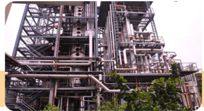
Distillation house & multi-effect evaporator
