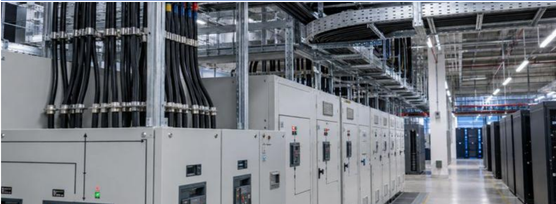
Next-Gen Data Centres Powering critical data centre in Hyderabad built by L&T, Sterling & Wilson, and Blue Star
