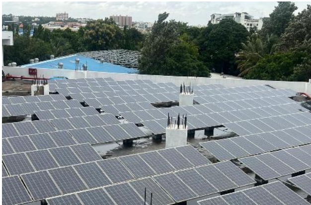
Solar Panel Projects continue with three more plants going live in FY24
