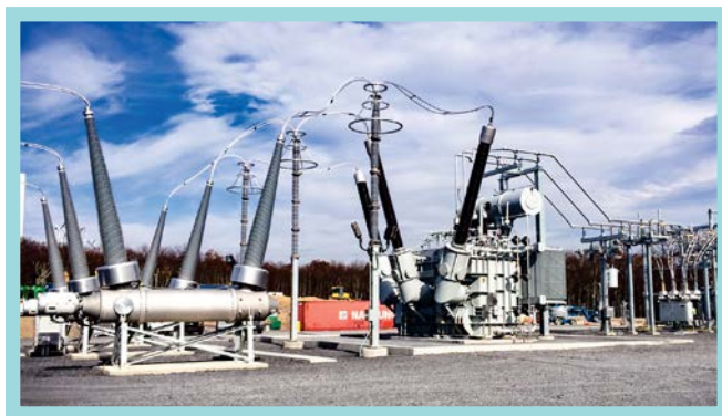
143 MVA 500 kV/34.5 kV/13.9 kV Power Transformer supplied for Wind Farm in the U.S.
