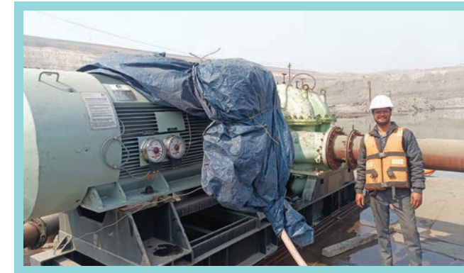
Commissioning activity of 900 kW 4Pole 6.6 kV HT Motors at Coal field in Nagpur
