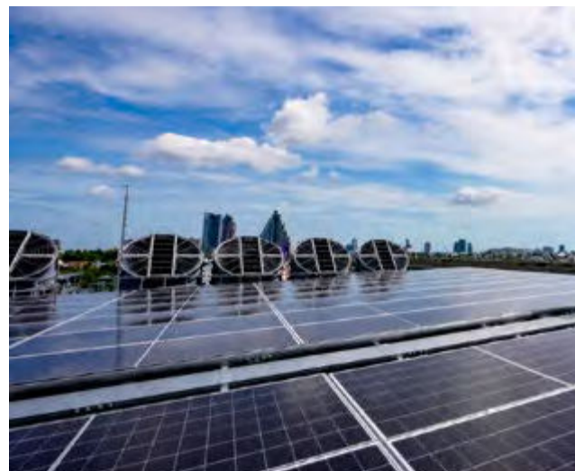
Rooftop Solar Panel
