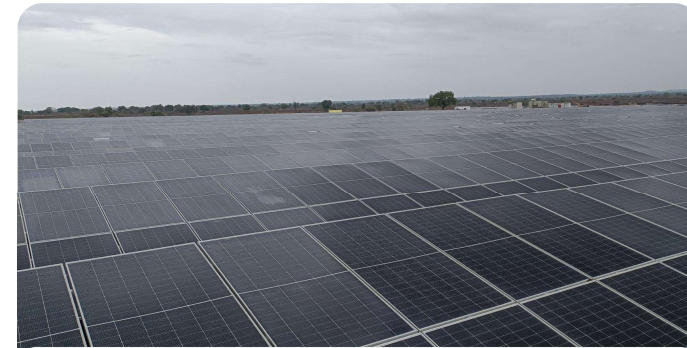
35 MWp Jalna, Maharashtra 1
