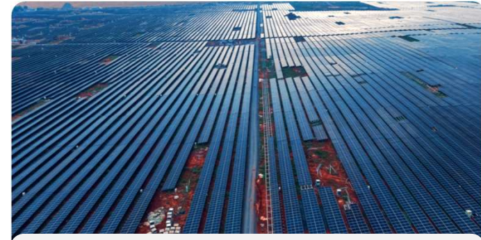
980 MWp Kurnool, Andhra Pradesh 1
