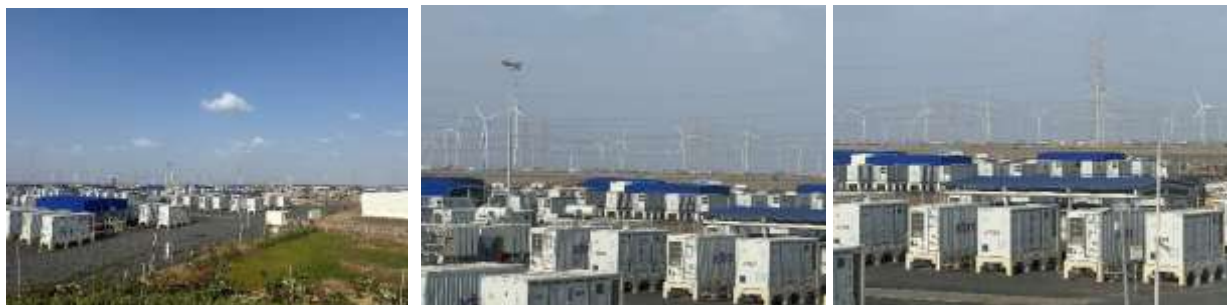
Photo: World's largest Battery Energy Storage at Khavda, Gujarat where Adani Green Energy is also developing the World's largest RE plant
