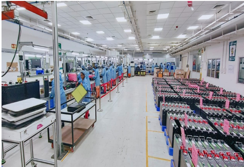
Pack Assembly Plant- Stationary- Divitipally Capacity ~ 1.2 GWh
