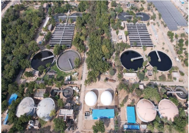
Upgradation of 50+50 MLD STP at Jodhpur, Rajasthan (includes solar and CBG plant)
