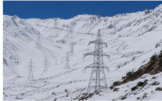
220 kV D/C Phyang-North Pullu T/L, Ladakh High altitude project
