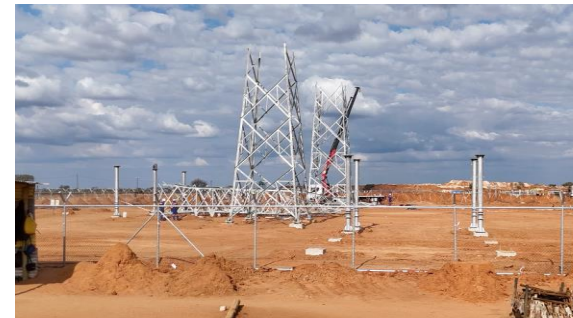
Mmamabula 400 kV substation, Botswana
