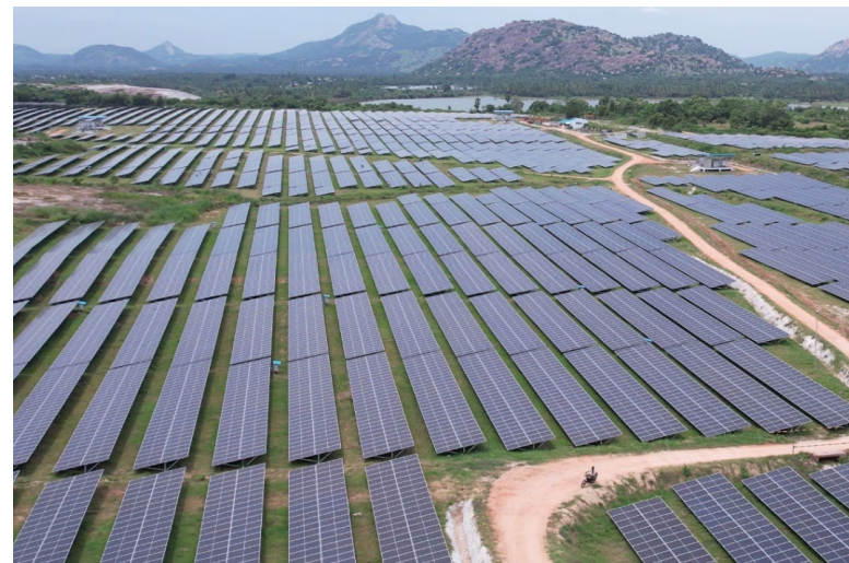
Solar panels (ground mounted)
