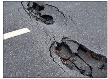
Damage is close where vehicles exit the expressway to connect with Karnal-Meerut highway.
