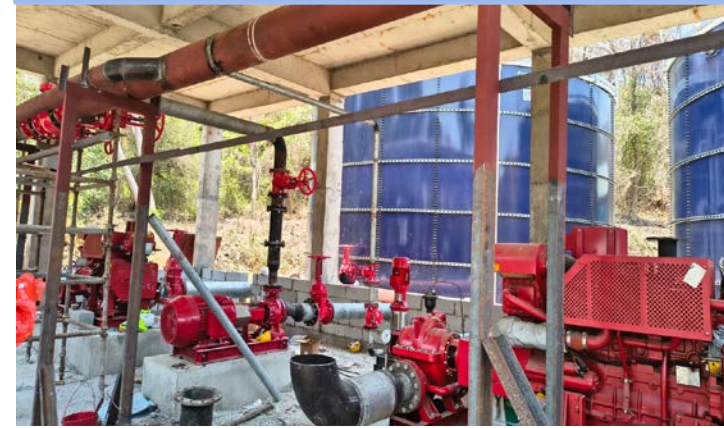
Fire Protection System – Mora – BA
