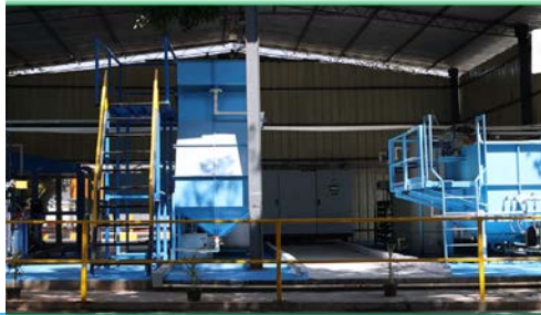
Electro coagulation for treating Effluent
