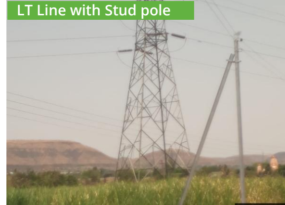
Danger board with Barbed wire
