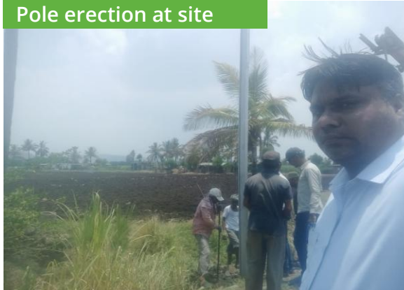
LT Line with Stud pole
