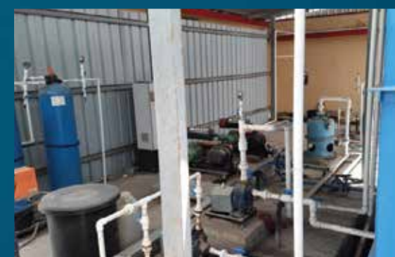
Water Conservation -STP Plant
