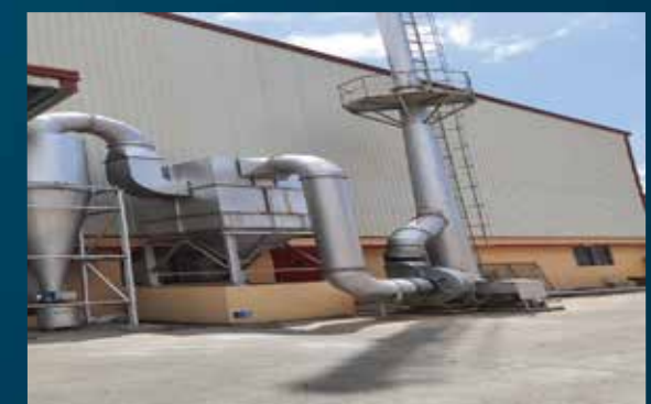
Waste Mangement -Dust Collector
