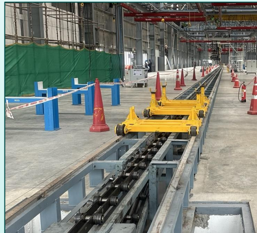
Conveyor Assembly Line
