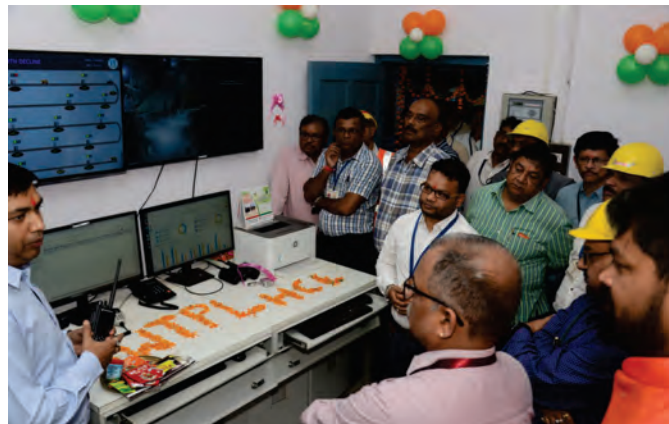
Underground leaky feeder-based communication system, installed and commissioned at Malanjkhand underground project for facilitating traffic movement and enhancing safety in the underground mine
