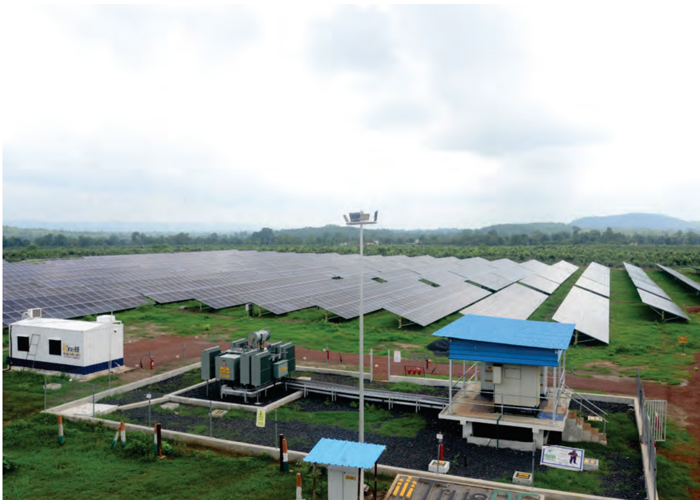
Solar Plant in MCP
