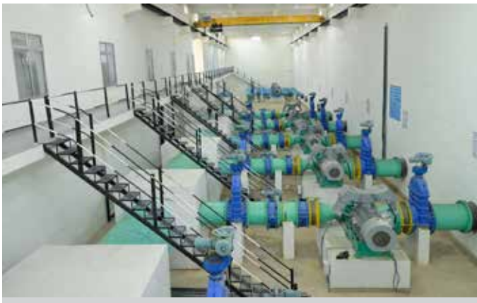
355 KW X 6 nos HSC Pumps at Balawala pump house in Bisalpur - Prithviraj Nagar Water Supply Project Phase-I Stage-I, Rajasthan.
