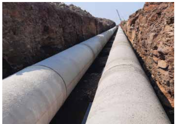
1700 mm dia PCCP pipeline laying for Jath Lift Irrigation Scheme, Sangli, Maharashtra
