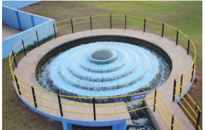
Cascade Aerator at Water Treatment Plant in Kandaila Multi Village Rural Water Supply Scheme in Rewa District in Madhya Pradesh.
