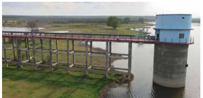
Approach Bridge constructed for a length of 588 meters and width of 4.20 meters at Intake well in Gadakota Multi Village Rural Water Supply Scheme in Sagar District in Madhya Pradesh.
