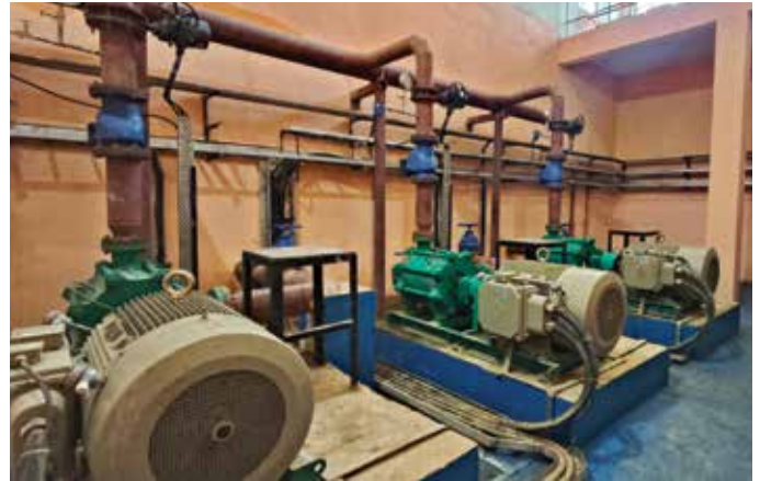
Installed HSC Pumps of Capacity 110 KW Each (2 Working + 1Stand by) at Intermediate Booster Pumping Station, Bhoopathi Laxmipur Village, Goribandha for Gajapati Water Supply Scheme, Odisha.
