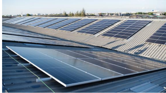
Rooftop mounted solar system
