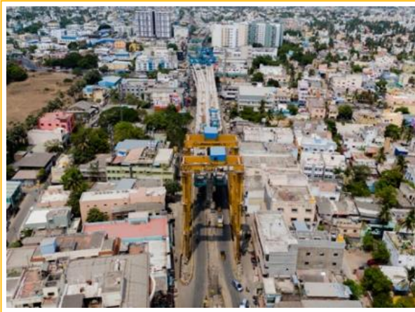
Chennai Metro [RMC supply]
