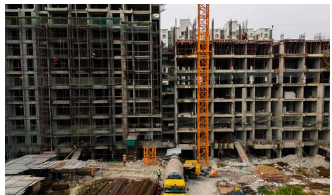
[RMC supply from Contract manufacturing plant in Turbhe, Mumbai]
