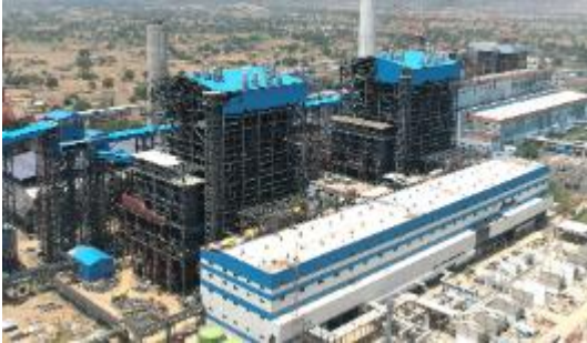
Unit #3 Turbine Bay Overview
