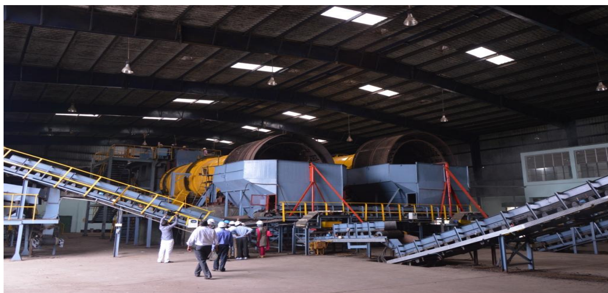
A view of ORSL's Solapur bioenergy facility, showcasing the company's technology and project execution capabilities.
