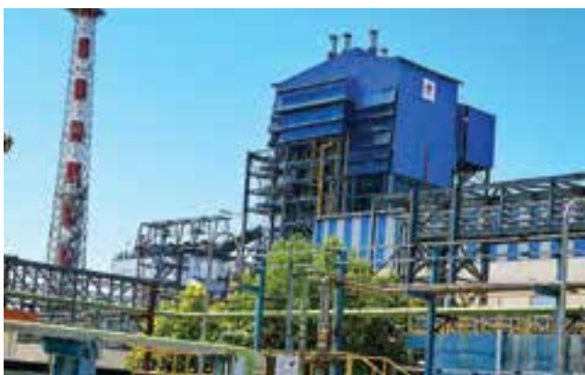
▲ CFBC Boiler Facility at Dahej.
