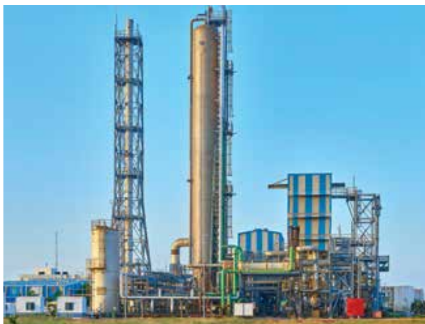
▲ Nitric Acid Production Facility at Dahej.
