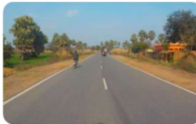
Upgradation of roads and bridges of Shivganj- Rafiganj-Goh-Uphara-Devkund-Baidrabad Road (SH-68, in the state of Bihar)
