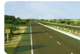
4 laning at Agra- Gwalior section, NH-2, in the State of Madhya Pradesh
