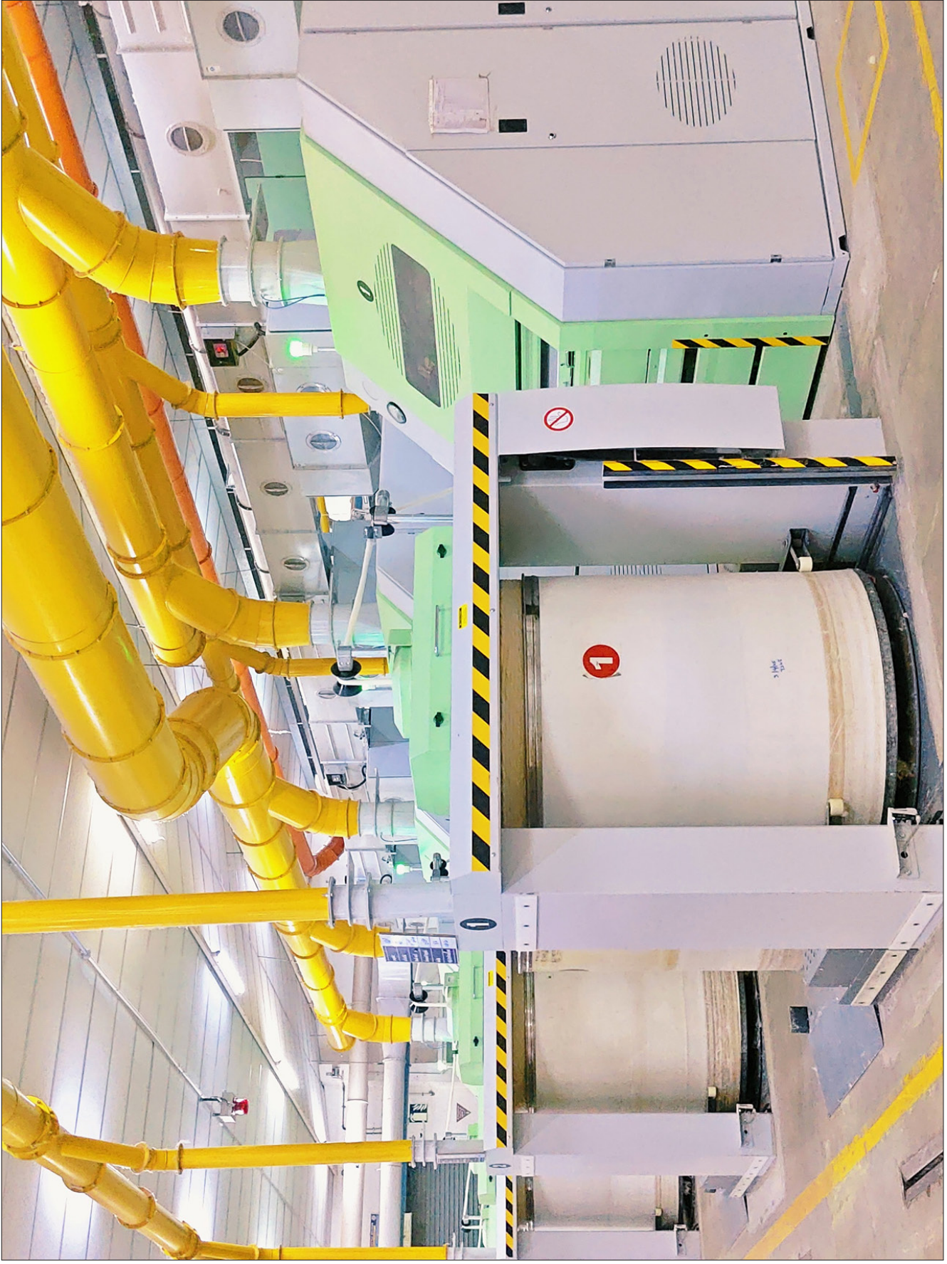
New LMW LC 361 S Carding Machine installed at C Unit in Sri Ramco Spinners.
