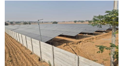
Solar Power Plant 3 Hisar, Haryana
