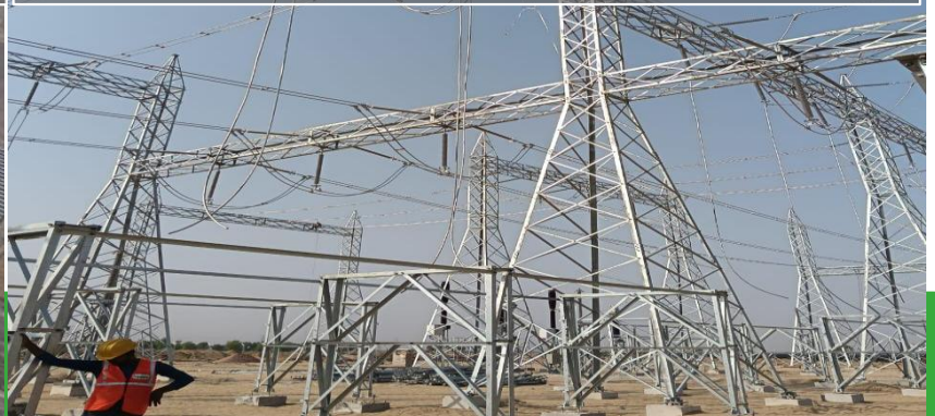
450 MWp Ground Mounted project at Bikaner, Rajasthan
