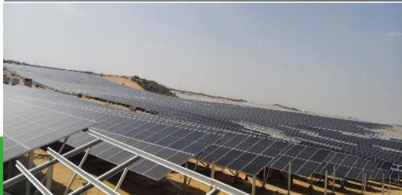
435 MWp Ground Mounted project at Bikaner, Rajasthan
