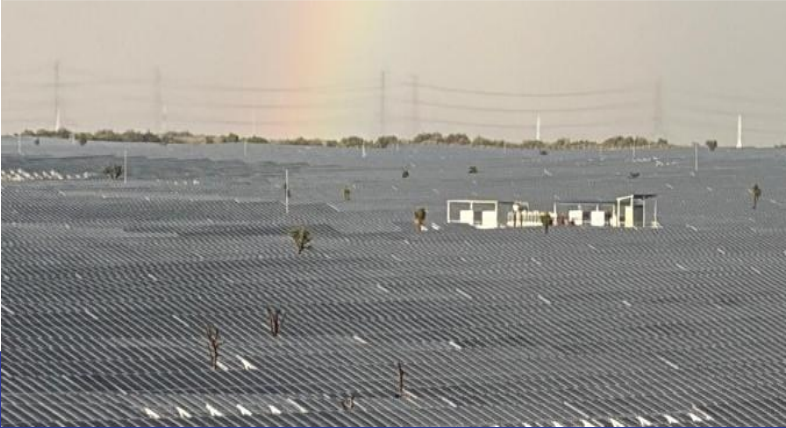
2012 MWp Ground Mounted project at Bikaner, Rajasthan
