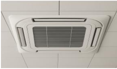
Cassette Air Conditioners (Ceiling-Mounted AC Units)
