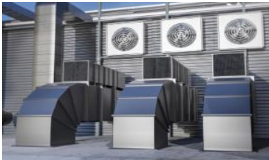
Industrial HVAC Systems / Air Handling & Ventilation
