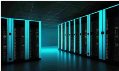
Data Centres / Server Room Cooling
