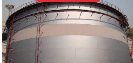
Floating Roof Tanks
